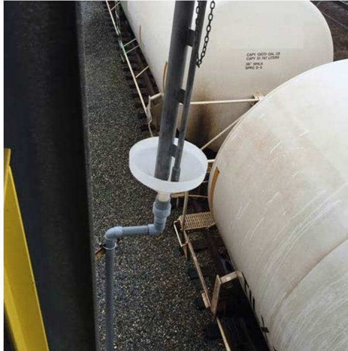
Image 16: Loading arm correctly placed in saddle to prevent spills to the environment
