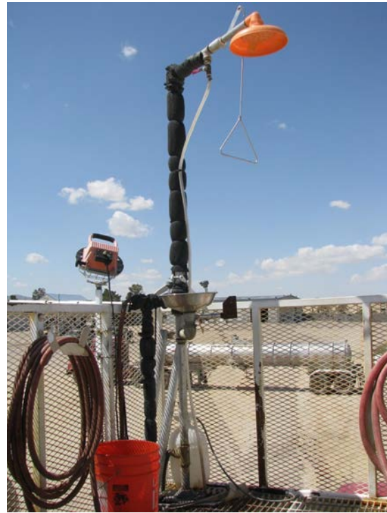
Image 8: Safety shower and eye wash station at transload rack
