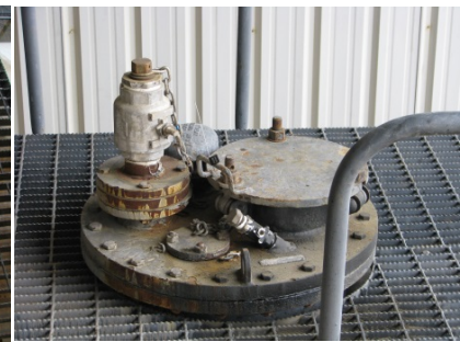
Image 5: No top fittings protection
