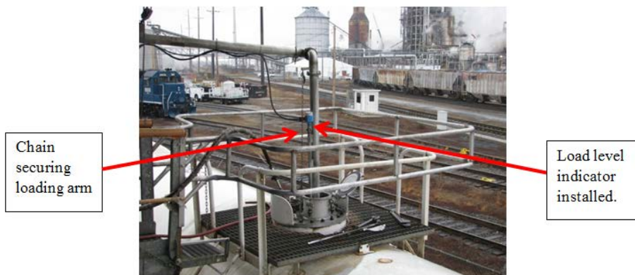
Image 15: Chain Securing Loading Arm & Load Level Indicator Installed
