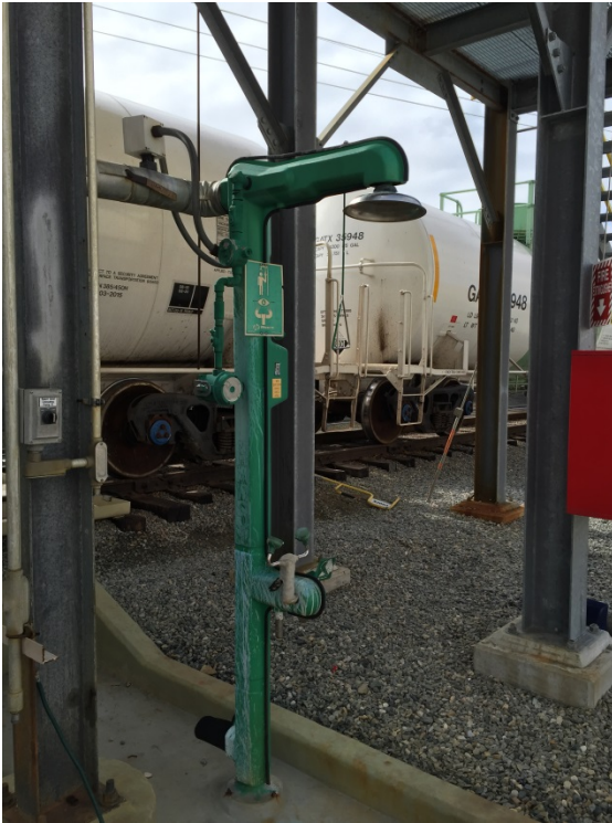
Image 7: Safety shower and eye wash station on ground level
