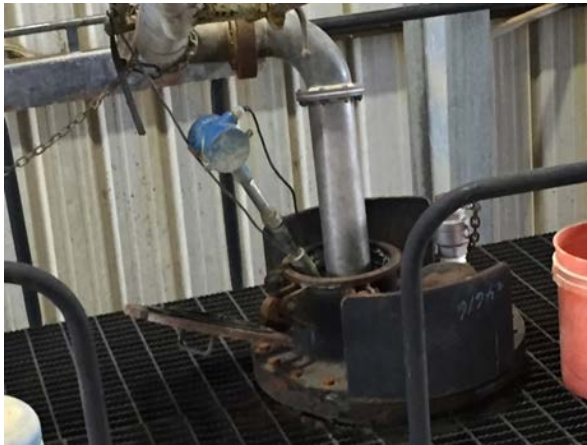
Image 1: Fill or load level detector installed for automatic shut off while loading through fill hole
