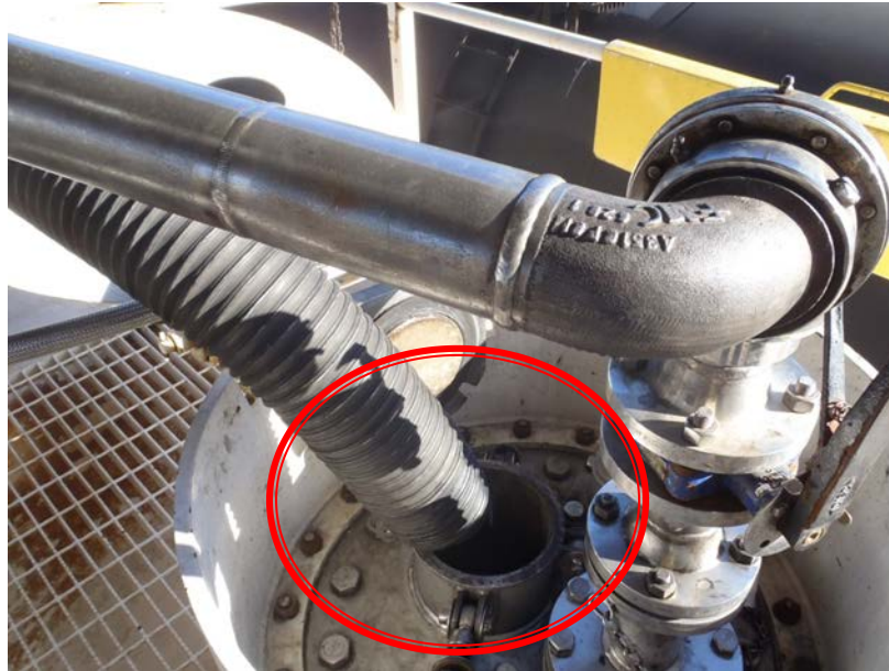
Image 24: Vent tube located above open fill hole to capture the gases of spent sulphuric acid
