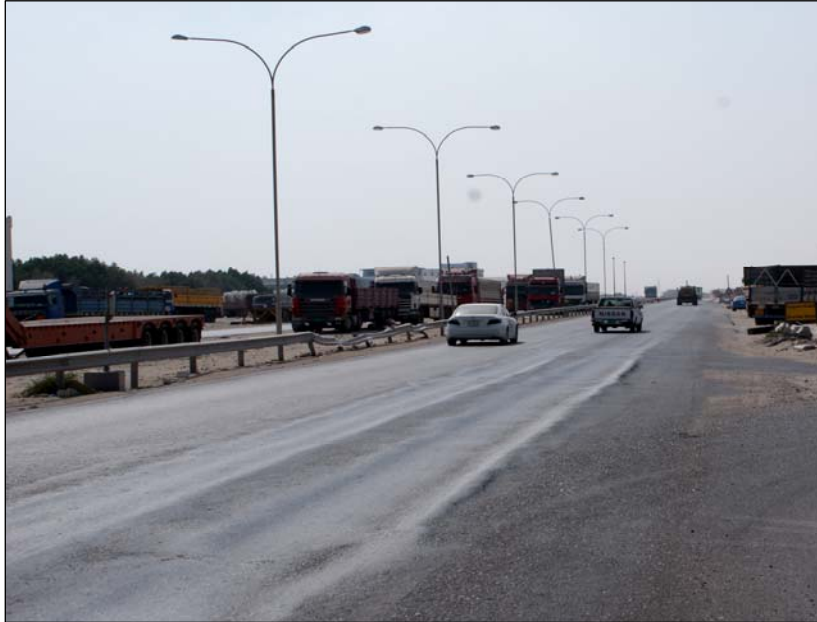
Figure 2: Permanent deformation in a road in Qatar.
