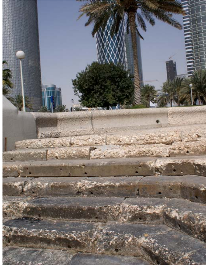
Figure 3: Portland concrete degradation from seawater, Arabian Gulf coastal area, Doha sea front (Corniche), Qatar.
